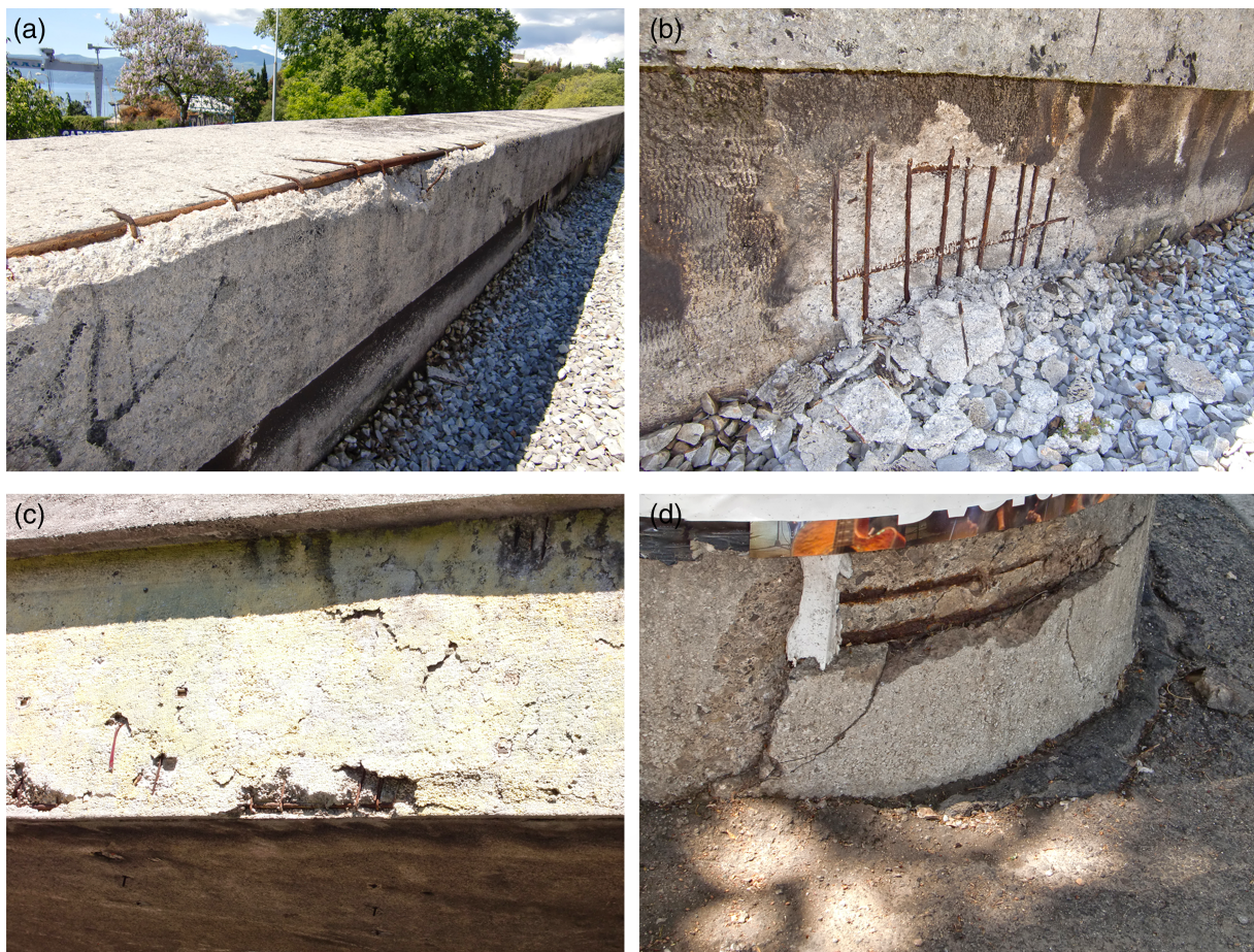
FIGURE 1 Concrete spalling caused by reinforcement corrosion: (a) Girder flange, (b) Girder web, (c) Slab, (d) Column
