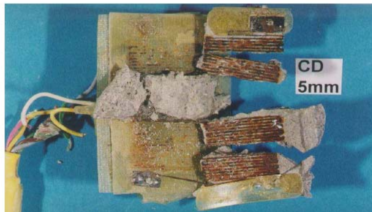
Legat, A. The Importance of Corrosion Monitoring for the Durability of Structures, Arches project
