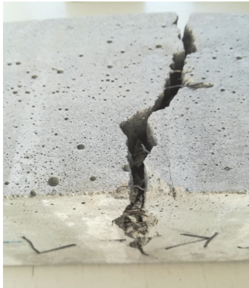
Figure 1. Steel fiber segregation in tensile zone of damaged beam
